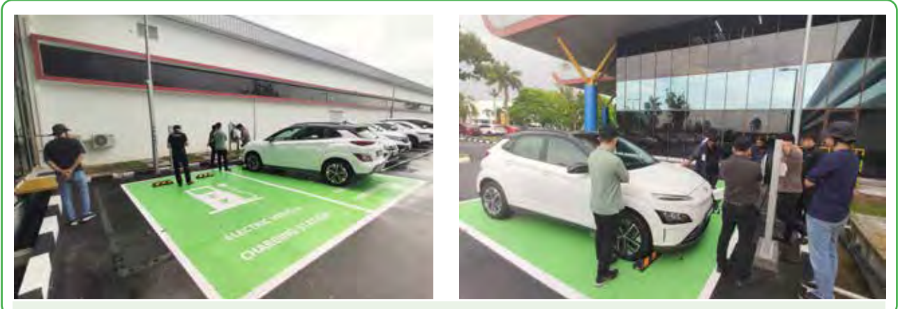
Installation of two EV charging stations at the parking area of BCM
